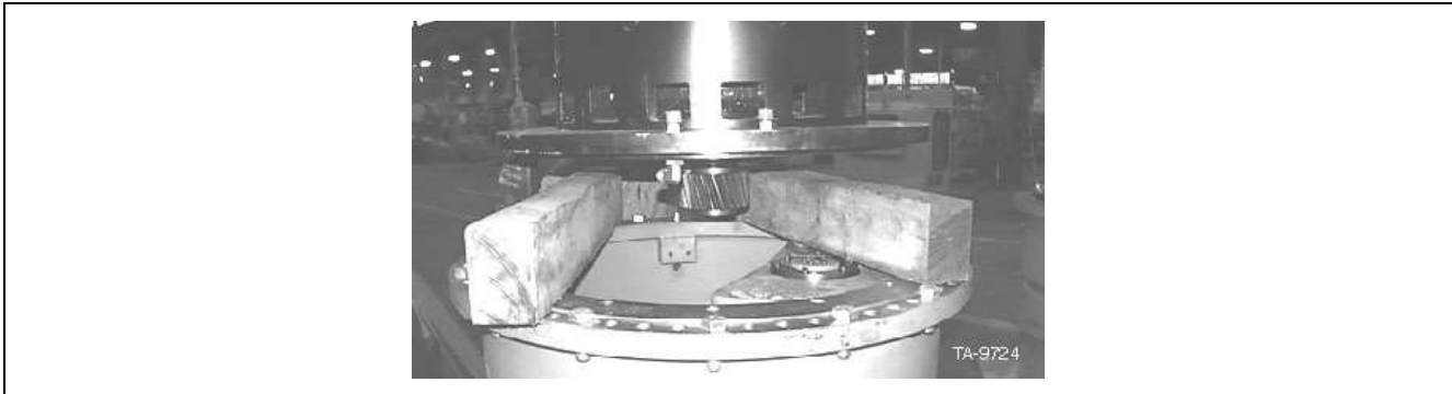
Figure 26. Blocking placed between planetary drive and traction motor for disconnection of oil return hose
