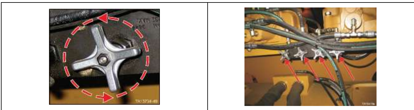
Figure 7. Pressure bleed down valves
