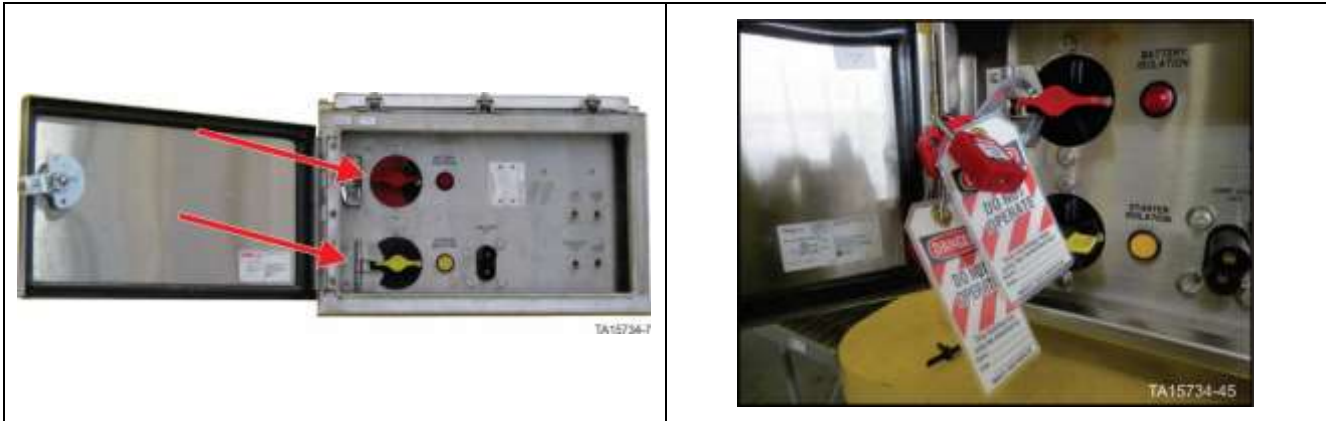
GEN 2 Battery Isolation Box – Battery isolation switch in OFF position with locks in place
