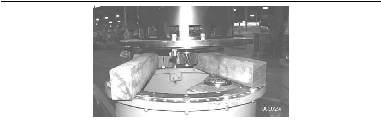
Figure 40. Blocking placed between planetary drive and traction motor for connection of oil return hose
