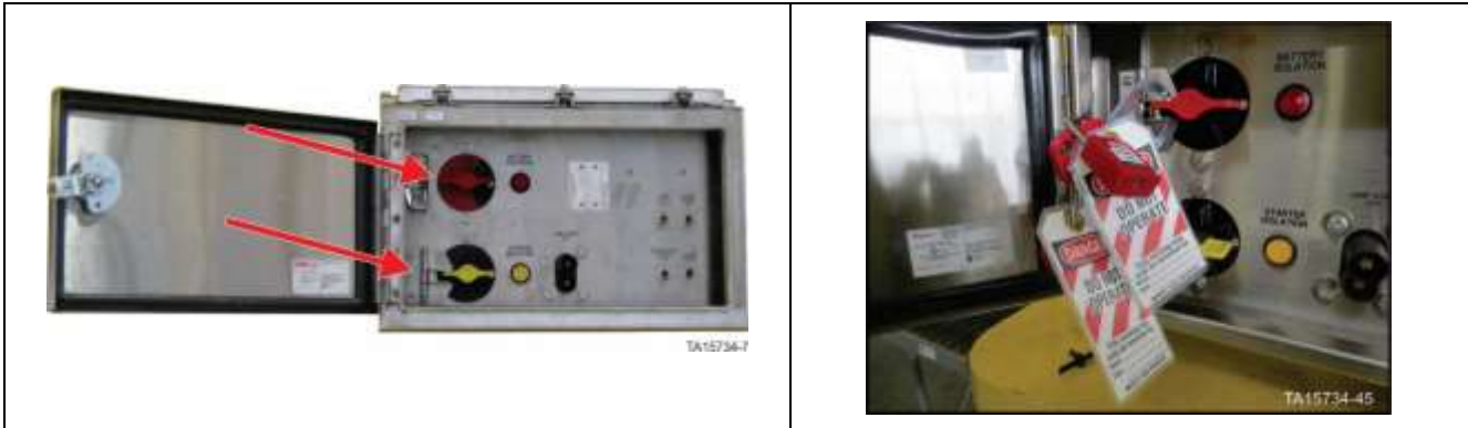
Figure 4. GEN 2 Battery Isolation Box – Battery isolation switch in OFF position with locks in place
